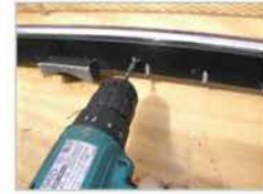
Install Step #15: With the Sport Grille removed drill for the remaining mounting screws and fasten all screws.
